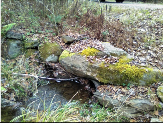
A culvert on a perennial stream in segment 170134 is undersized, posing a risk of washing out and causing erosion downstream.
