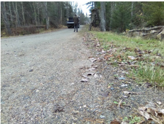
Road shoulders in all segments are above the surface of the road, requiring reshaping to shed water as sheet flow. The road surface is not crowned enough to shed water effectively.
