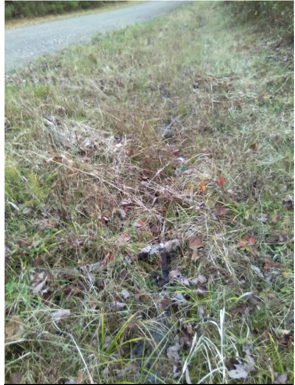
Steep segments in segment 170133 lack stone lining in ditches, causing erosion.
