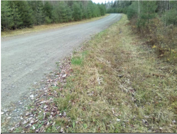
Steep ditch segments in segment 170134 require stone lining.
