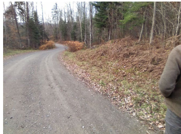
Shallow ditches need to be reestablished in segment 170135 and 170136. Precautions will be taken to not spread the knotweed present.
