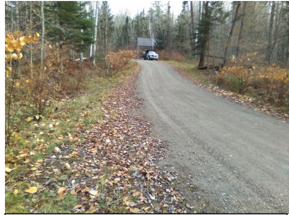
Steep ditch segments in segments 170135 and 170136 require stone lining.
